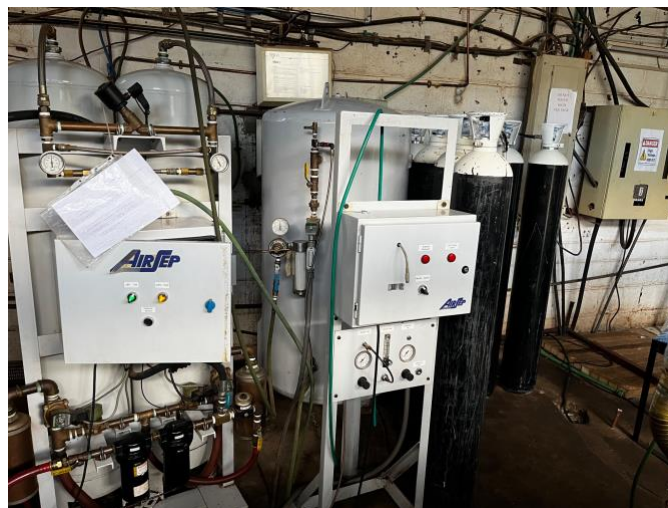
A hospital's oxygen concentrator. Note that this size machine is not sufficient for the hospital's needs- the tanks on the right side are connected in-line to the system and changed as needed, to add to the system's capacity.
