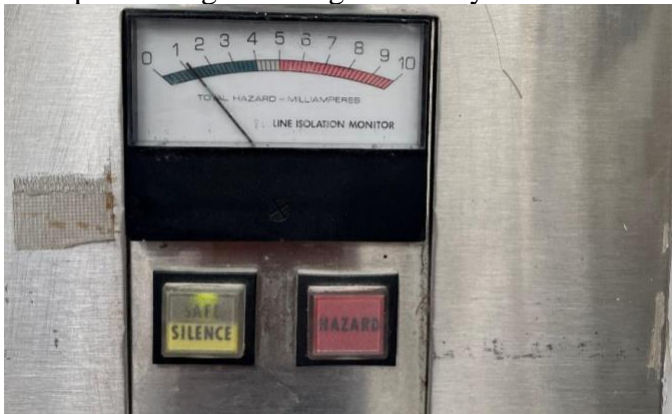
A Line Isolation Monitor in a resource-rich hospital.
