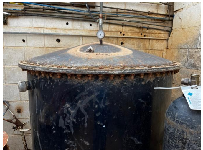
The buffer tank of the same system as above, with a pressure gauge that can easily be checked to confirm that the system is working properly.
