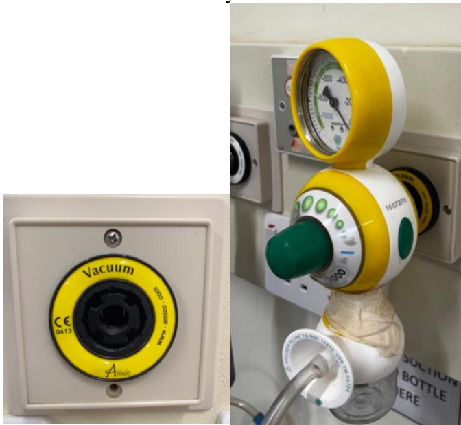
A wall connection for medical vacuum, unconnected (left) and connected to a regulator (right). Other brands or types of regulators cannot be used with this system.
