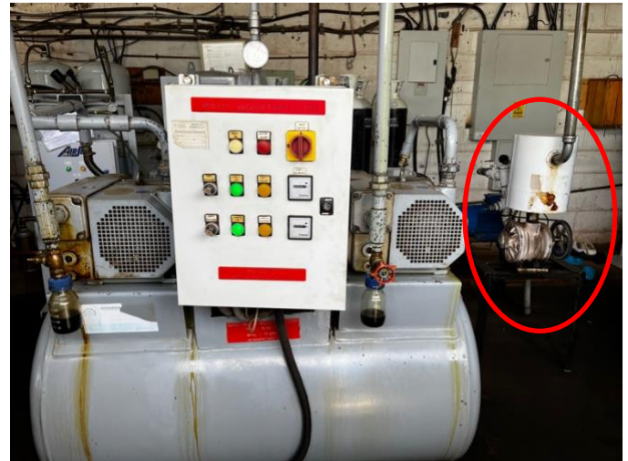
Centralized vacuum system in a hospital in a resource-limited setting, with a control panel in the foreground and a back-up system in the background (Red circle.)
